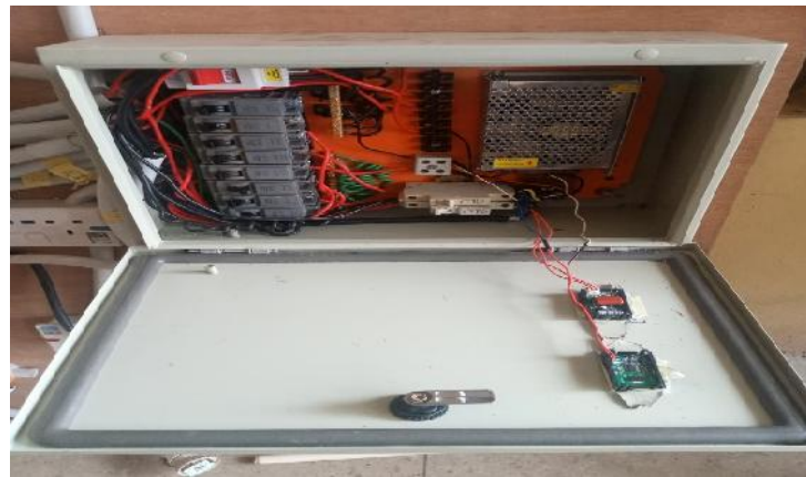
Figure 3: Hybrid Consumer Unit Showing Inner Construction.
