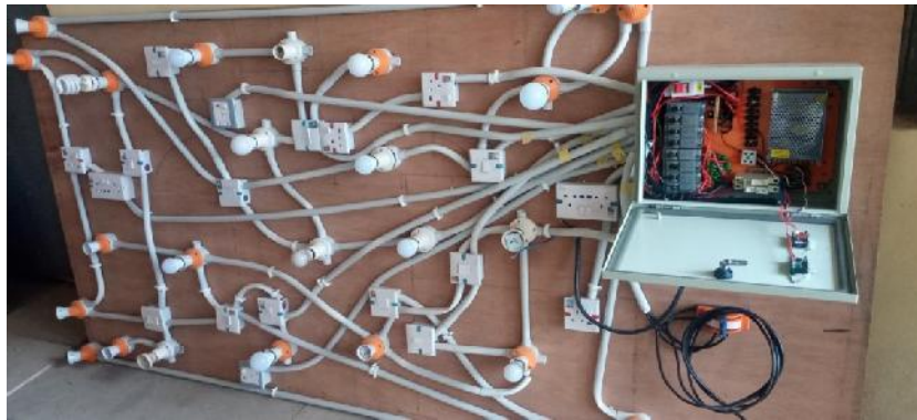
Figure 4: Hybrid Consumer Unit Supplying Power to the Prototype Three-Bedroom Apartment.
